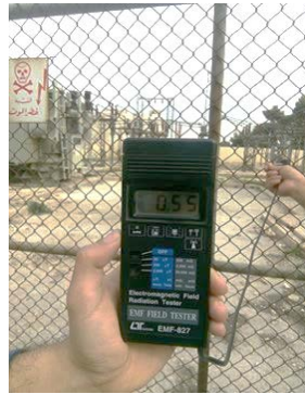
Fig. 3: Reading EMF on the fence of a substation
