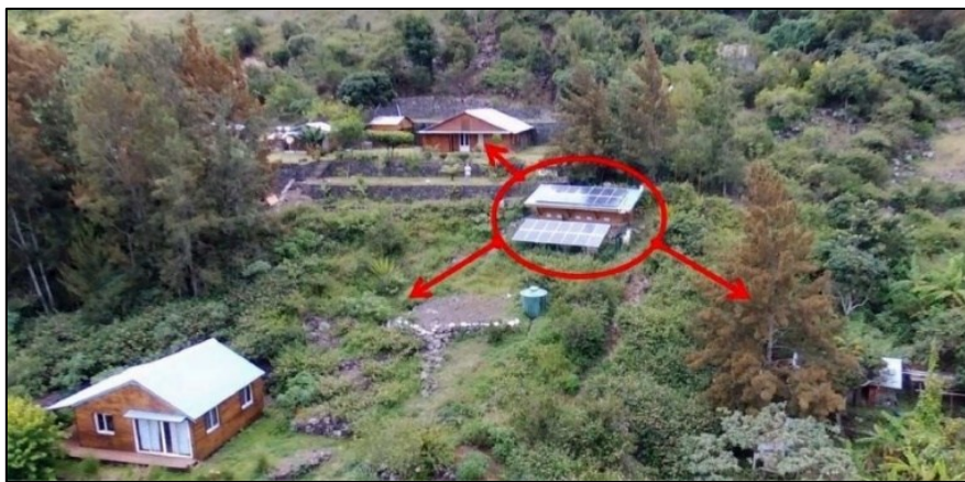
Fig. 1. Aerial view of the microgrid showing the battery pack and the acquisition devices at the center, with the loads positioned at each of the three ends [16].
